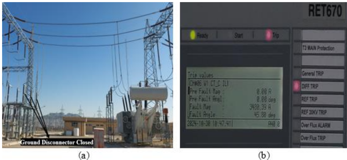
Figure 2: (a) Applying a short circuit by closing the earthing switch at the T3 output. (b) Measuring the contact current by the protective relay
