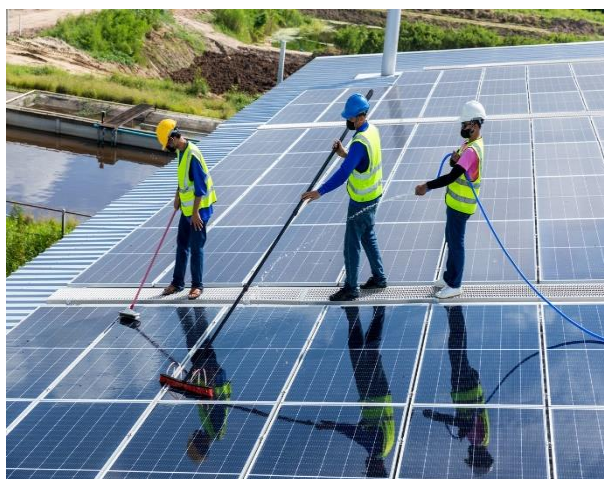
Figure1.3: Manual Solar Panel Cleaning Process
